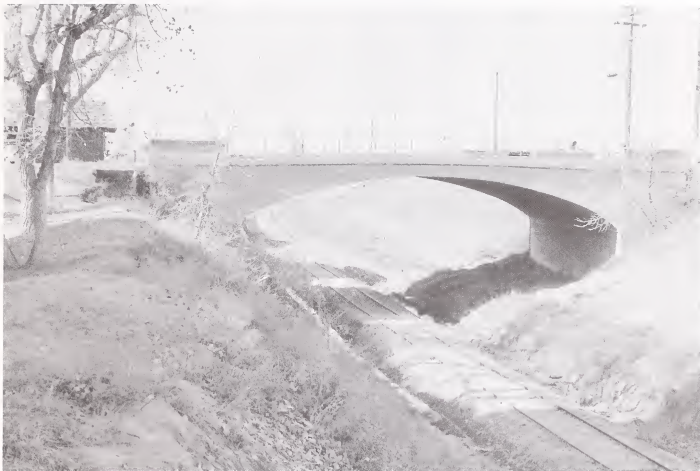
The CMSTP&P Railroad Overpass in Great Falls was one of several road-related reinforced concrete structures built by the company during its early years in the state.
